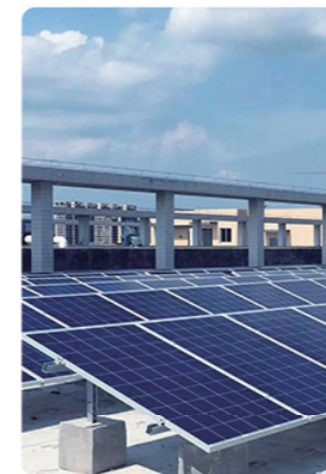
PHOTOVOLTAIC ENERGY STORAGE
